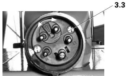
Fig. 39: Electricity socket with phase inverter
